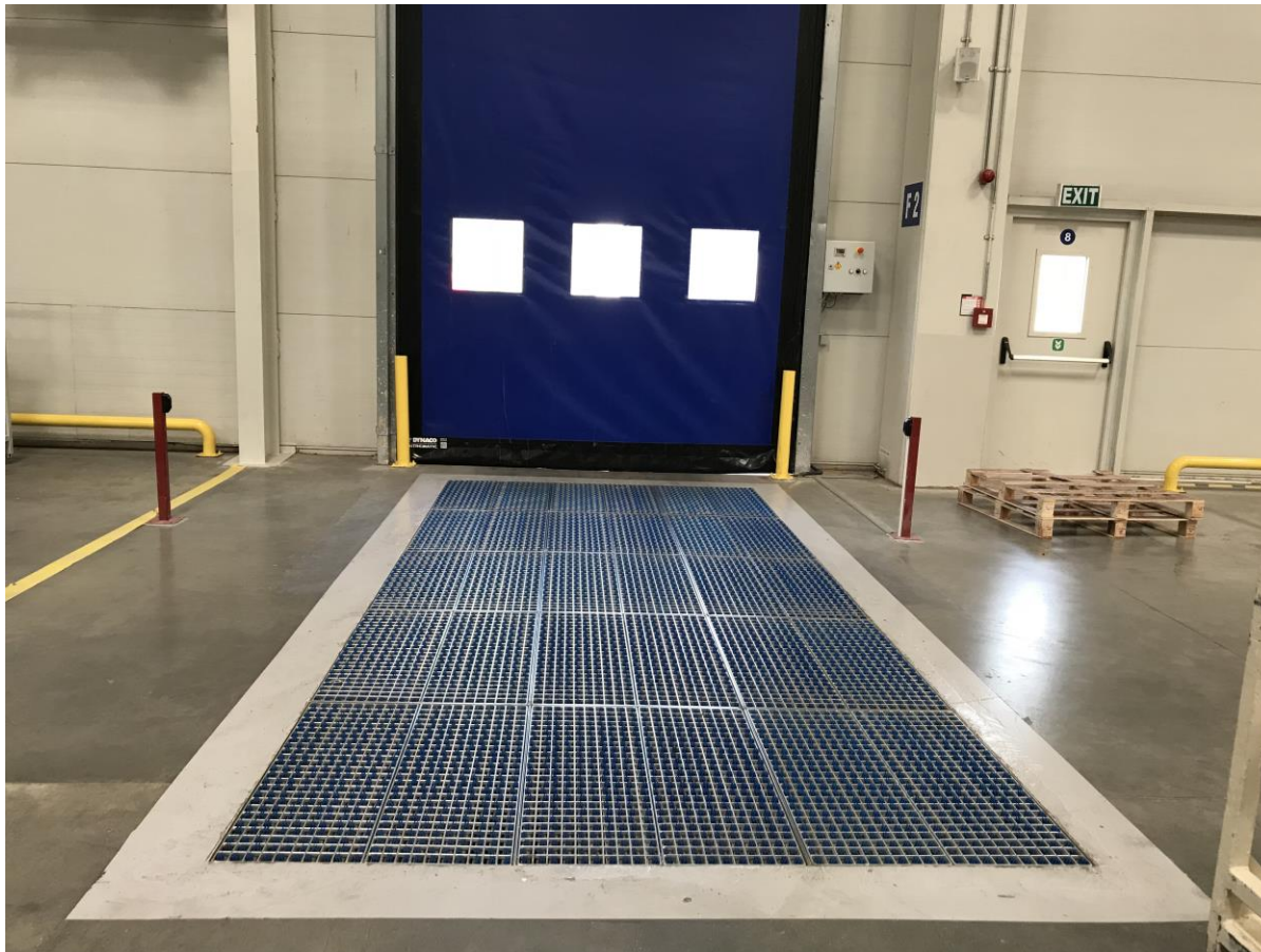
Second installation at factory in Kocaeli
